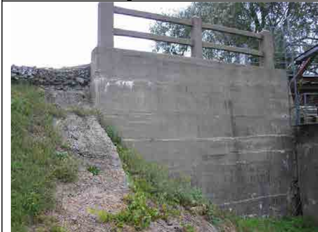
Photo #11 – Right downstream wingwall. Note the seepage at the interface between the wingwall and right most downstream pier.
