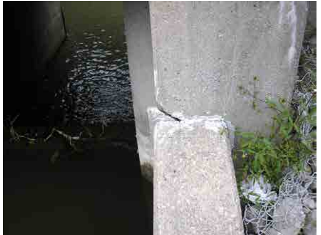
Photo #20 – Right upstream wingwall, looking downstream. Wingwall movement responsible for deterioration of right abutment concrete.
