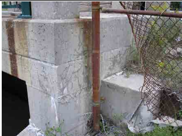
Photo #21 – Alkali silicate reaction above the right upstream wingwall. Sheet pile evident, in line with stop logs. Opening in fence. Alkali silicate reaction.
