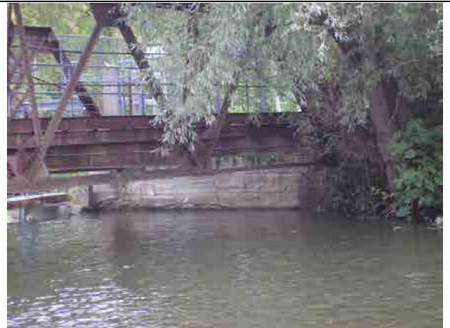
Photo #16 – Close up view of the right upstream wingwall. Concrete spalling observed at the waterline, and extends along length of wingwall.
