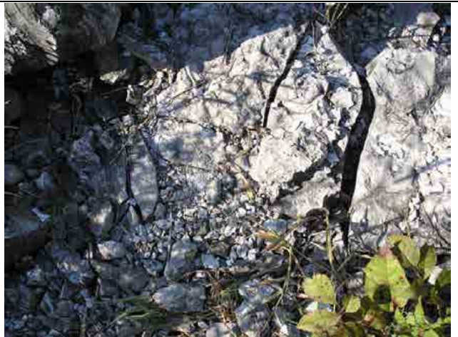
Photo #6 – Close up view of the deterioration of the riprap along the slope of right upstream embankment. Riprap varies from 10 to 1000 mm.
