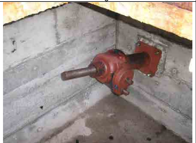
Photo #10 – Lift mechanism inside lift chamber used to open and close the low flow gate located. LPRCA staff reports lift mechanism is functioning properly.
