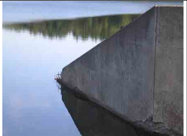
Photo #20 – Left upstream wingwall, as seen from the right upstream bank. Note concrete spalling at the waterline.
