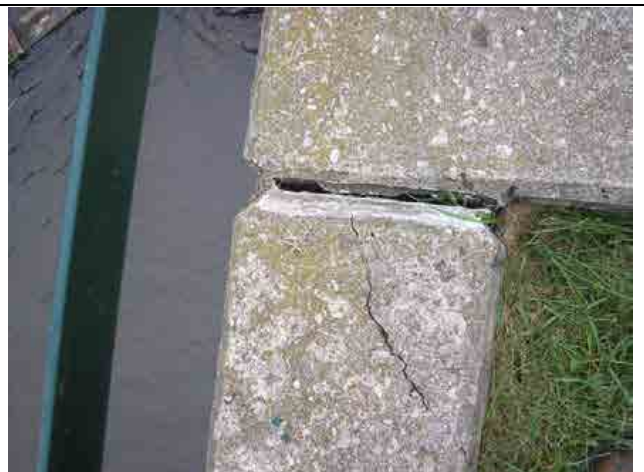
Photo #42 – Crack and joint movement at the right downstream wingwall and fish ladder channel structure.
