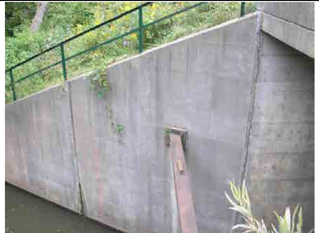
Photo #26 – Right downstream wingwall. Note the steel brace installed to limit lateral movement between downstream wingwalls.
