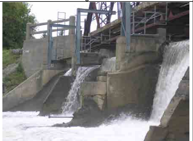
Photo #40 – Teeterville Dam piers. Note the heavy concrete deterioration at the base of the piers.
