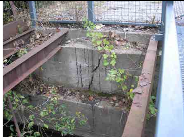
Photo #27 – A crack at the left upstream wingwall, below the old roadway surface.
