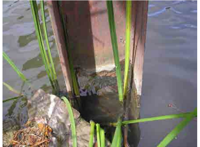
Photo #32 – Left bent. Corrosion through the web observed at waterline.
