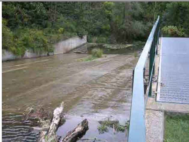
Photo #33 – Lehman Dam main spillway, standing on top of wingwall and looking downstream.
