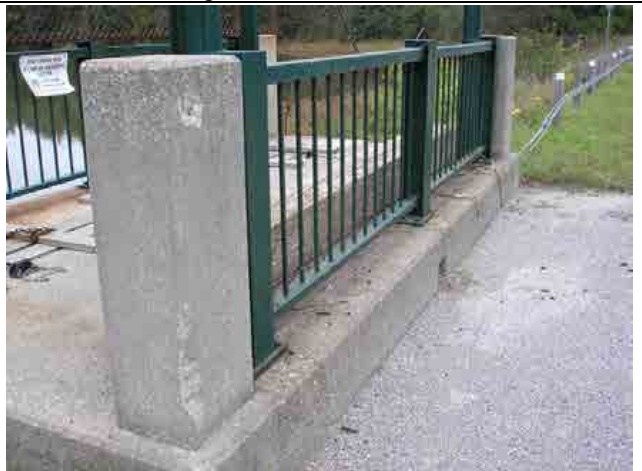
Photo #22 – Minor deterioration (spalling) of concrete adjacent to the railing on the upstream side of the bridge.
