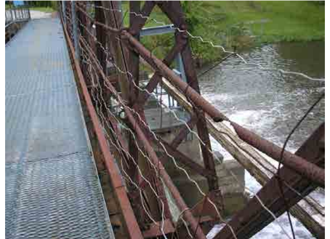
Photo #32 – Railing at the bridge is loose, and consists partially of fence wire.
