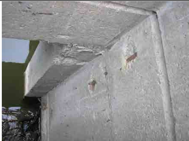
Photo #17 – Exposed reinforcing bar above left gain, looking down from deck.
