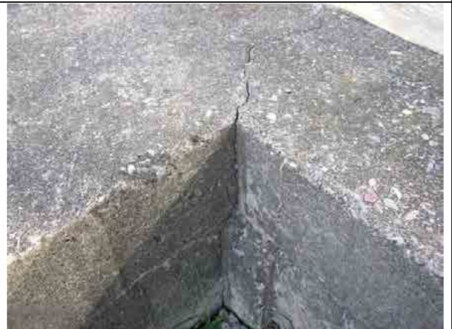
Photo #24 – Same crack on the wetwell-wingwall interface, isometric view.
