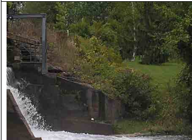
Photo #17 – General overview of the left downstream wingwall, seen from the right bank. Seepage through the wingwall at the left bank was observed.
