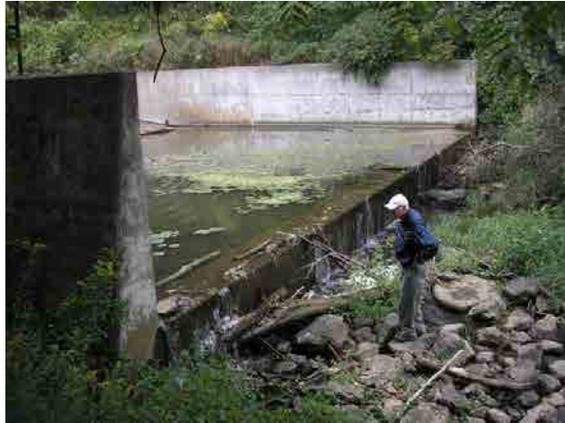
Photo #37 – Stilling basin and downstream channel. Note the missing riprap stone downstream.
