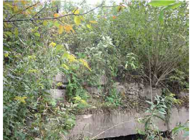
Photo #20 – Close up view of the slope above right downstream wingwall. Vegetation is growing through the grouted concrete blocks.
