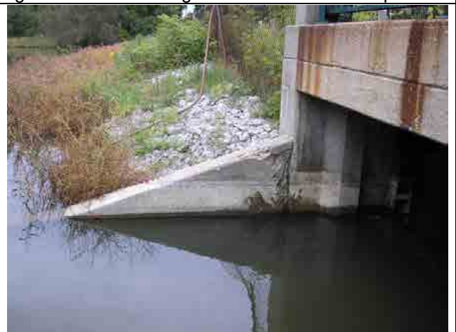
Photo #12 – Concrete deterioration at the left upstream wingwall.
