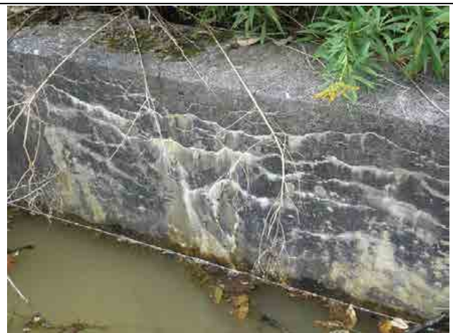
Photo #48 – Low flow outlet structure, left downstream wingwall. Note alkali-silica reaction.
