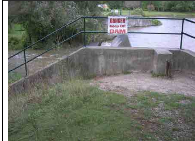
Photo #37 – Left downstream wingwall note localized fill erosion.
