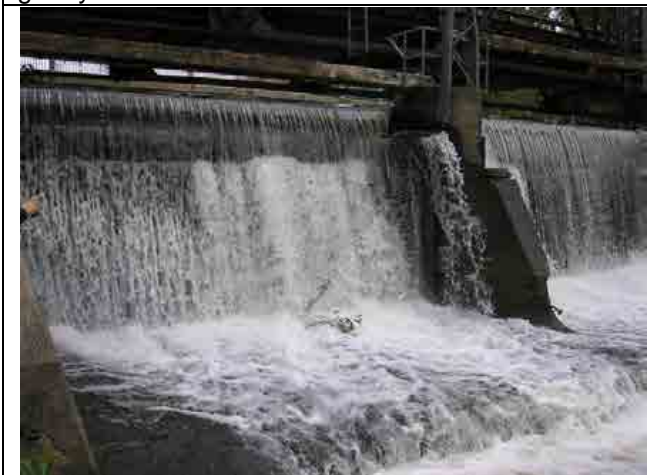
Photo #41 – Right most bay; concrete at the piers heavily deteriorated.
