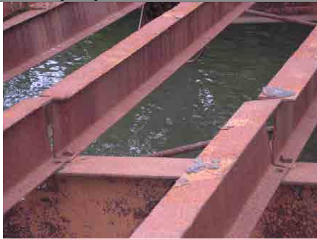
Photo #33 – Majority of the stringers spanning the girders are out of alignment.
