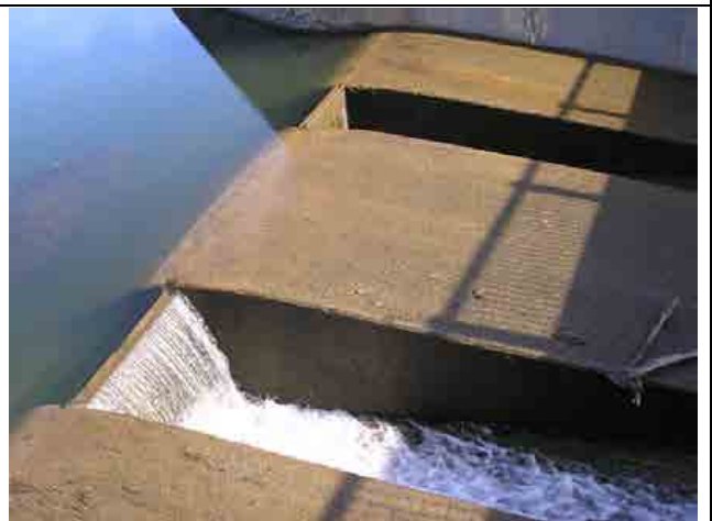
Photo #40 – Main spillway, as seen from the right bank. Top right stop log has shifted and is allowing more water to spill.
