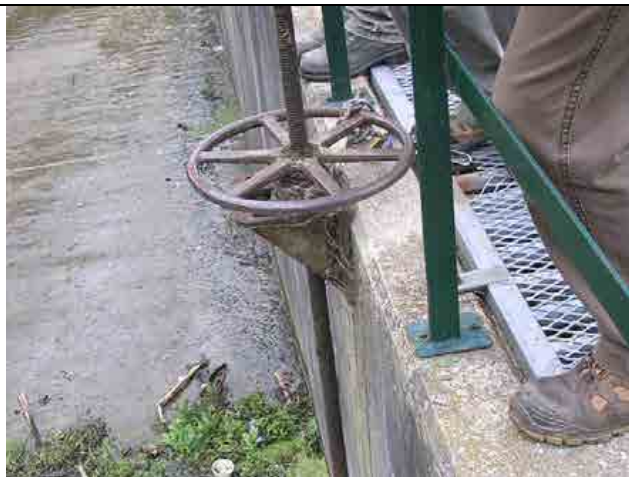
Photo #35 – Fish ladder intake gate in the right upstream wingwall. LPRCA staff informs gate is functional.
