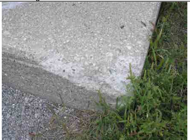
Photo #24 – Close up view of minor concrete spalling on the downstream pad.
