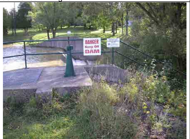
Photo #18 – Wetwell at right wingwall. Gate not tested during inspections. LPRCA staff notes gate is functional.
