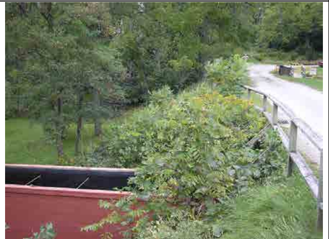
Photo #16 – Left downstream embankment, looking towards the main spillway. Note tree and brush vegetation on and adjacent to the slope.
