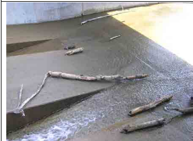
Photo #41 – Main spillway, underneath the road bridge. Note debris on the spillway.
