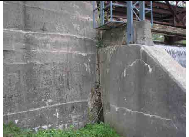
Photo #12 – Close up of the seepage through concrete at the interface between the wingwall and right most downstream pier. Note concrete deterioration in wingwalls and pier.
