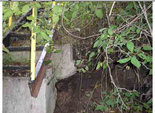
Photo #24 – Left downstream embankment left of the access stairs consists of slope that is over steepened. Localised loss of embankment fill was observed.
