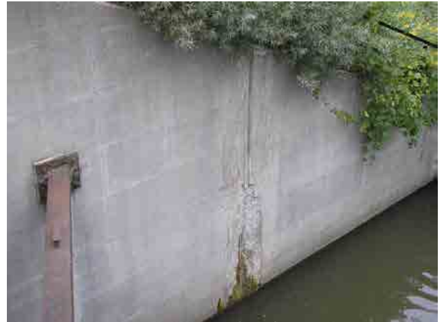
Photo #32 – Left downstream wingwall, downstream most section. Note seepage through joint.
