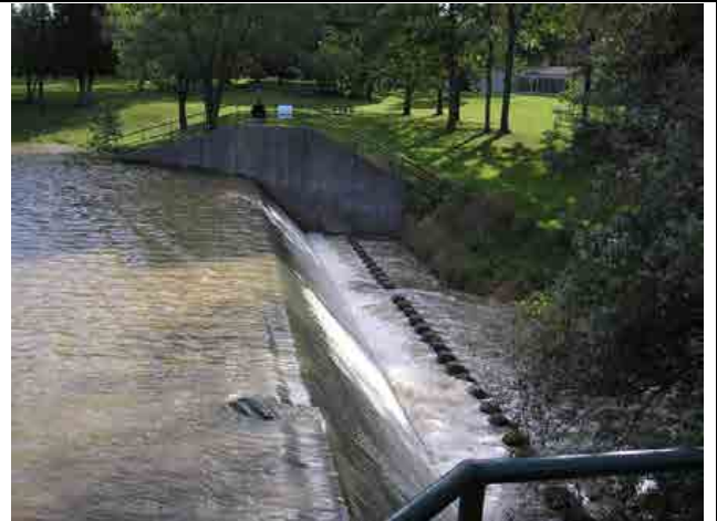
Photo #14 – Norwich Dam main spillway and stilling basin. Note minor damage to some of the baffle blocks.
