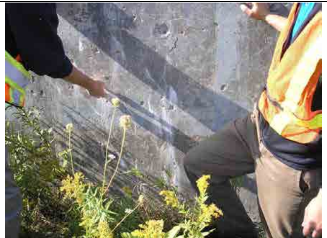
Photo #18 – Some amount of alkali-silicate reaction on top of the left upstream wingwall.
