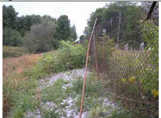
Photo #6 – Left upstream embankment, standing at left wingwall looking towards left. Gabion mattress adjacent to left upstream wingwall. Damaged fence.
