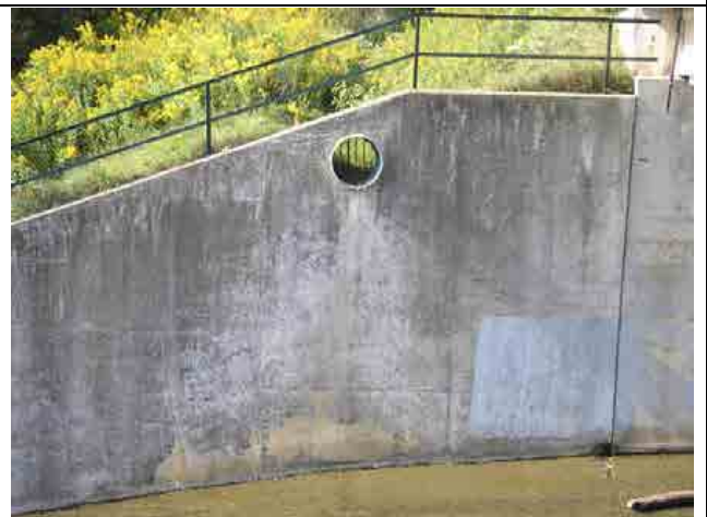
Photo #34 – Right downstream wingwall, panel 1. Panels are numbered from 1 (at bridge) to 8 (at spillway). No joint filler material between panels.
