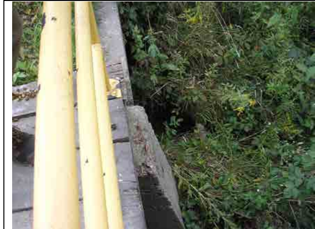
Photo #25 – Void in the left downstream embankment noted, adjacent to the left downstream wingwall.
