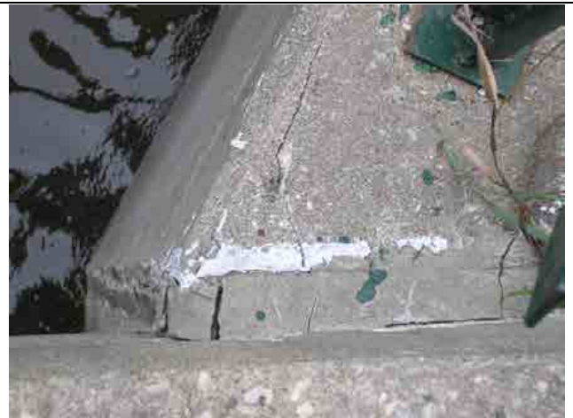
Photo #30 – Joint movement at right downstream wingwall.
