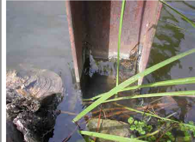
Photo #31 – Right bent. Corrosion through the web observed at waterline.
