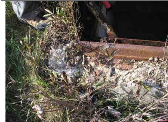
Photo #13 – Close up view of the concrete spalling outside of the lift chamber.
