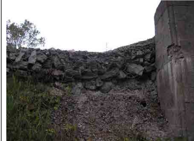
Photo #13 – Gabion mattress located on top of the right embankment at the right downstream wingwall. Downstream slope appears grouted; holes in the grout are observed.
