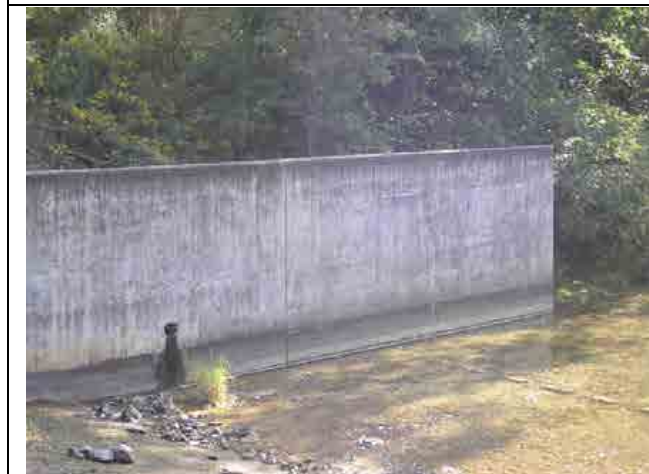
Photo #33 – Left downstream wingwall, panel 8. Corrugated steel toe drain noted as functional.
