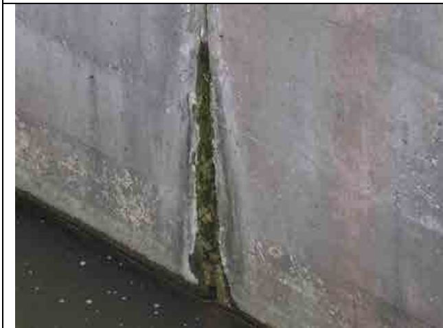
Photo #27 – Joint at right downstream wingwall. Wetness and moisture at the joint indicates backfill material is no longer free draining and water is building up behind the wall.
