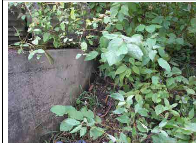
Photo #21 – Wetness was noted adjacent to the bank-wingwall interface, at the left downstream wingwall.
