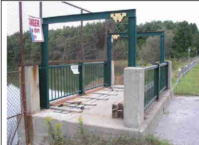
Photo #3 – Hay Creek Dam control structure, with stop log lifting frame.
