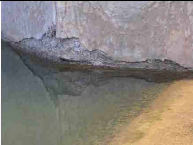
Photo #21 – Close up of the concrete spalling at the waterline.
