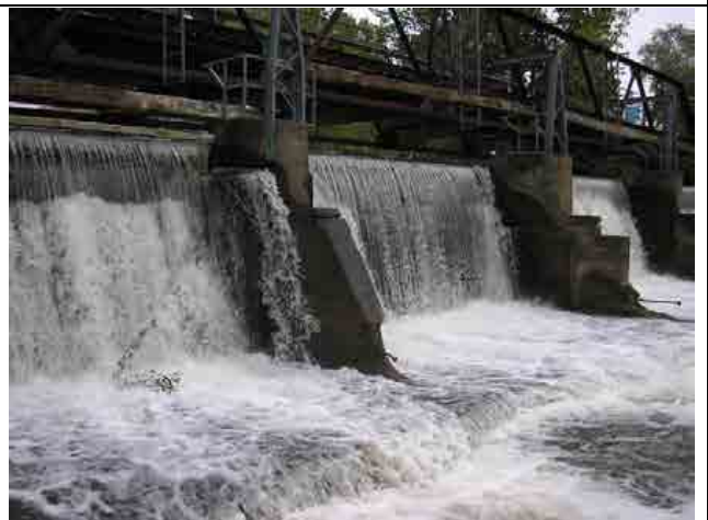
Photo #42 – Concrete is also heavily deteriorated at the inner bays of the dam. Note the elevation difference between the sill of the dam and the bottom of channel.
