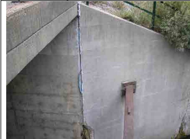
Photo #33 – Upper portions of the joint between bridge abutment and left downstream wingwall. Note exposed joint filler material and seepage below.
