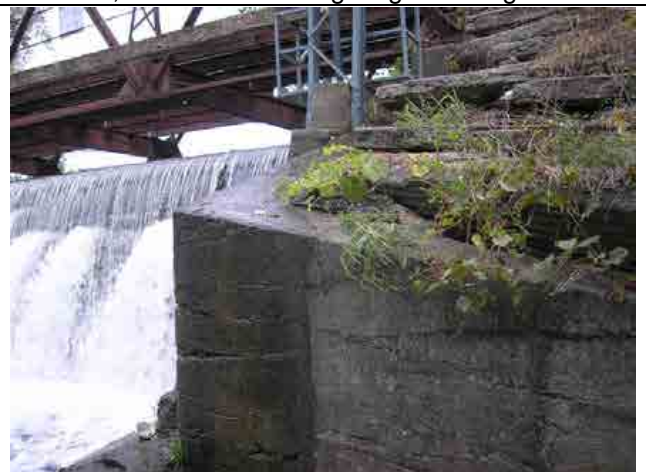
Photo #18 – Left downstream wingwall. The seepage noted was between the left most pier and the wingwall concrete.
