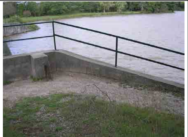
Photo #36 – Left upstream wingwall. Note localized fill erosion adjacent to wingwall.
