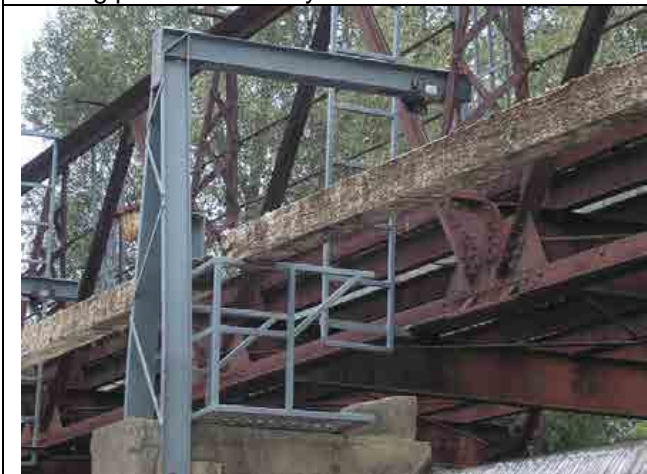
Photo #39 –Gantry crane as seen from the left bank. Note that stop logs are resting on the hand rail of the gantry crane.
