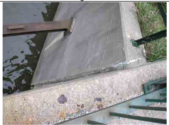
Photo #28 – Top view of the joint at the interface of the bridge abutment and right downstream wingwall. Most of the lateral movement is at the top.
