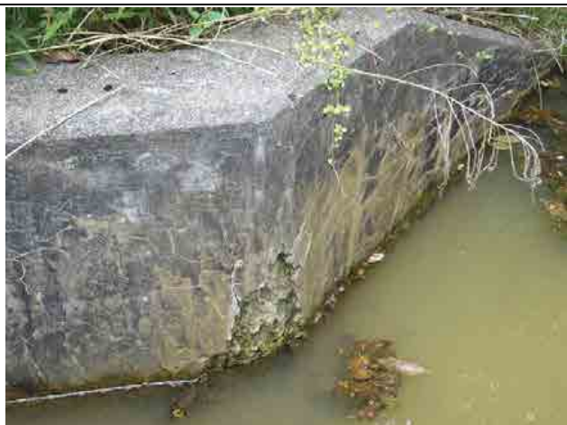
Photo #47 – Low flow outlet structure, left downstream wingwall. Note concrete deterioration.
