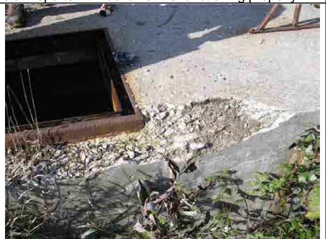
Photo #12 – Concrete spalling on the outside of the lift chamber. Damage likely exacerbated from application of salt during winter on adjacent road.
