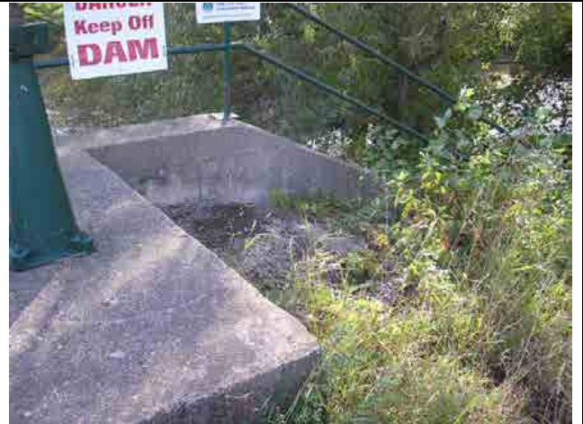
Photo #20 – Handrail at right downstream wingwall. Top surface of embankment downstream of wetwell is surfaced with asphalt.
