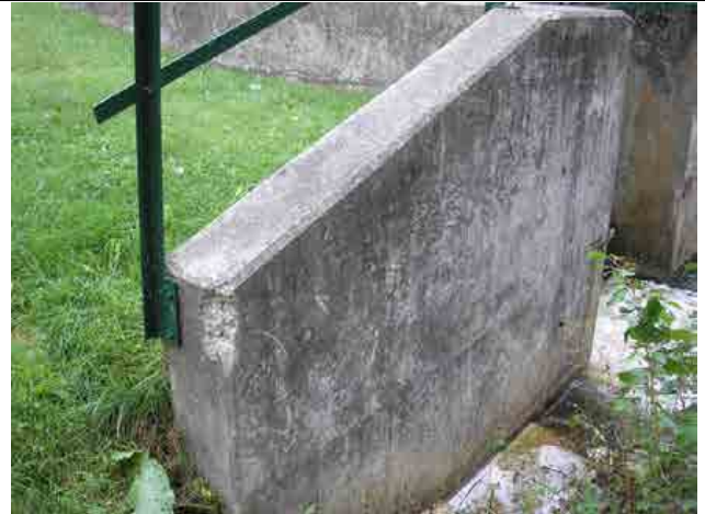
Photo #10 – Right wingwall of the outlet structure. Minor spalling of concrete on the downstream side. Concrete is generally in good condition.
