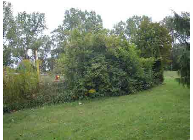
Photo #10 – Upper portions of the left downstream embankment. Seepage, cracks or loss fill through left embankment were not observed.
