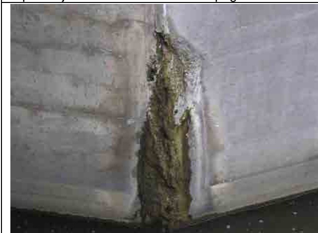
Photo #35 – Close up of the joint between bridge abutment and left downstream wingwall. Moisture along wall indicates water build up behind wingwall.
