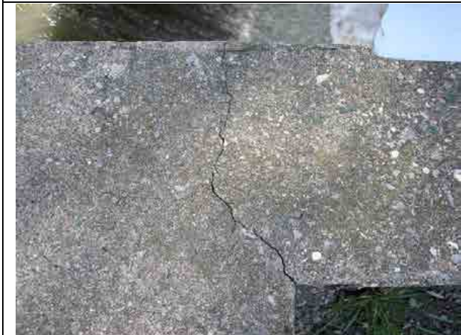
Photo #23 – Top view of the crack at the wetwell-wingwall interface, on the downstream face.
