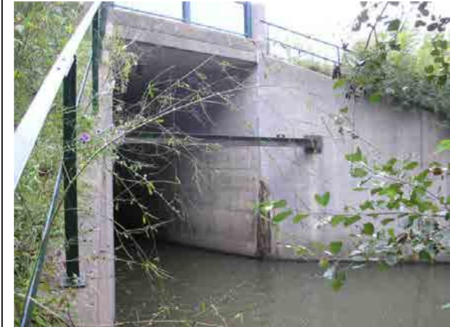
Photo #31 – Left downstream wingwall. Note horizontal brace and seepage through joint between wingwall and bridge abutment.
