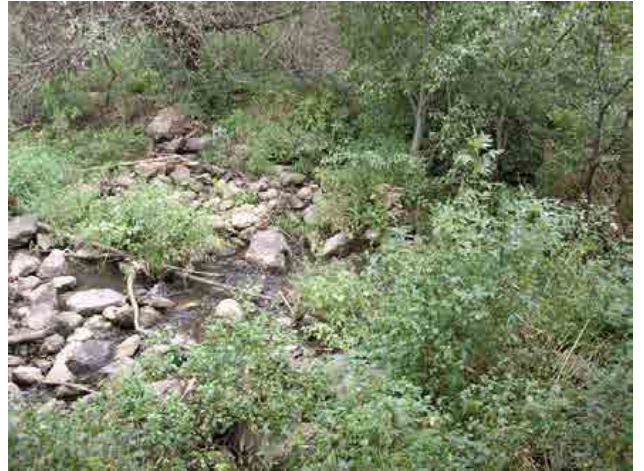
Photo #38 – Channel downstream of the spillway is heavily vegetated with brush. Loose riprap evident.
