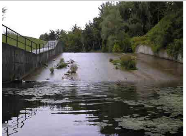
Photo #34 – Main spillway, standing in stilling basin and looking upstream. Minor vegetation growing through the concrete spillway observed.
