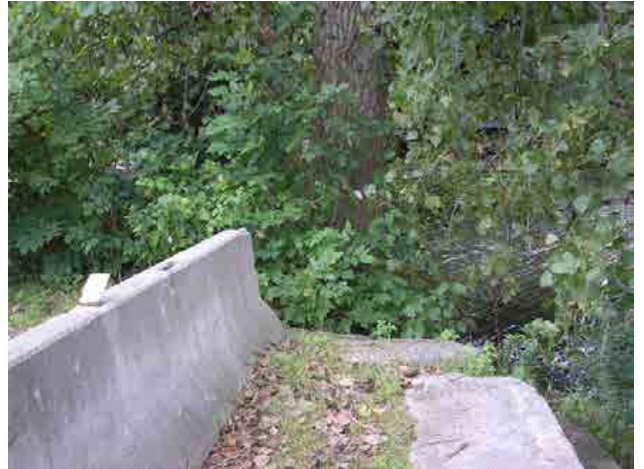
Photo #26 – A mature tree is growing at the left upstream wingwall, adjacent to the old steel truss.
