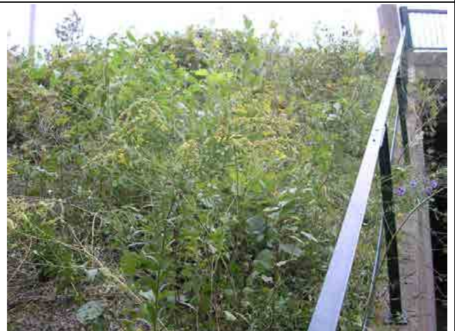
Photo #10 – Right downstream embankment, looking towards road. Portion of the embankment adjacent to right downstream wingwall is surfaced with asphalt.
