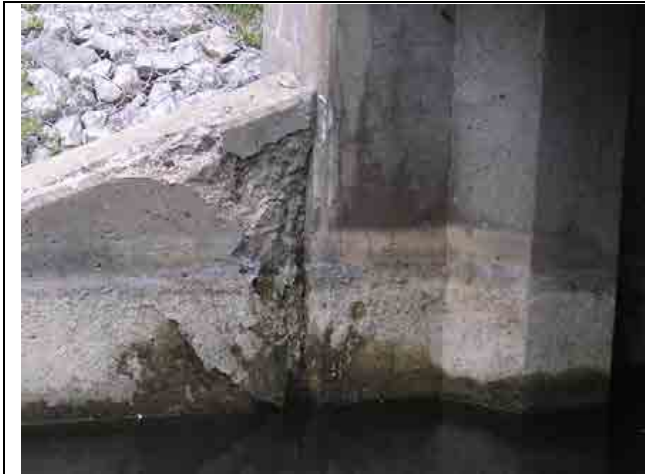
Photo #13 – Close up of the deterioration at the left upstream wingwall.
