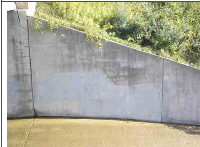
Photo #29 – Left downstream wingwall, panel 1. Panels are numbered from 1 (at bridge) to 8 (at stilling basin). No joint filler material between panels.
