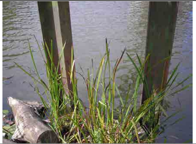
Photo #30 – Bottom of the pile bent, at the waterline.
