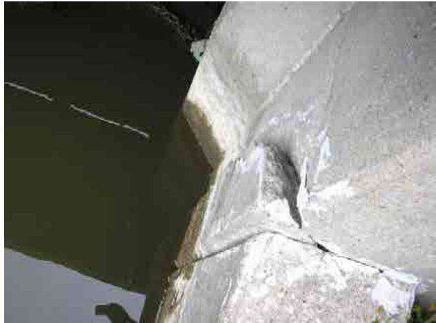
Photo #19 – Movement evident in the right upstream wingwall.
