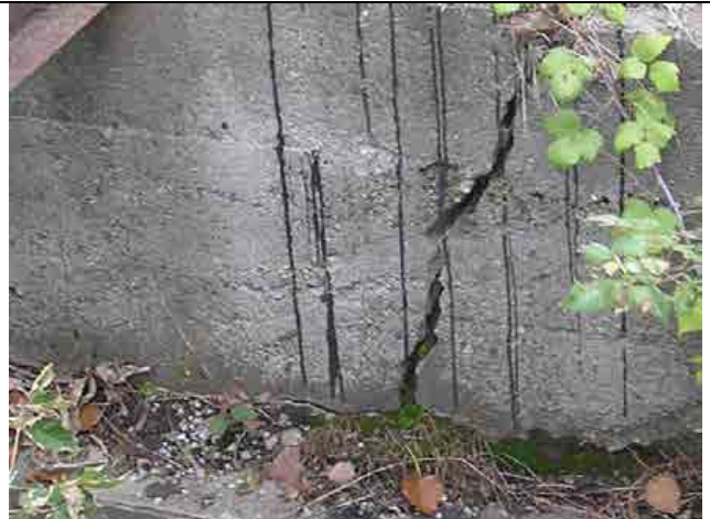
Photo #28 – Close up of the crack at the left upstream wingwall. Width of the crack is in excess of 10 mm.
