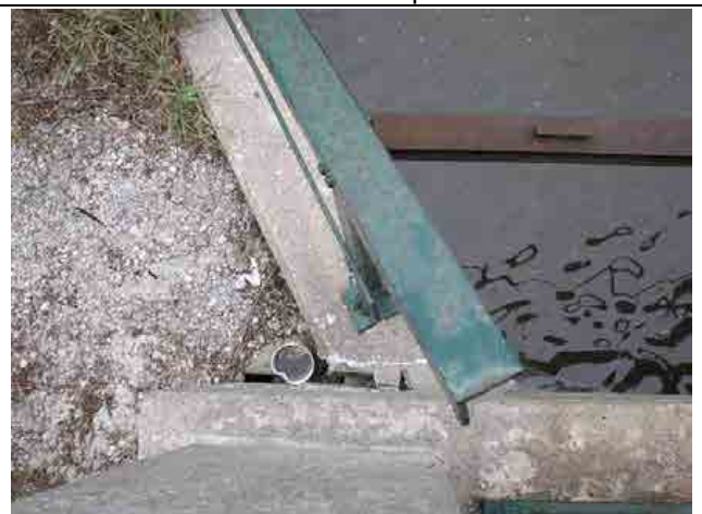
Photo #36 – Top view of the joint between bridge abutment and left downstream wingwall. Note joint movement.
