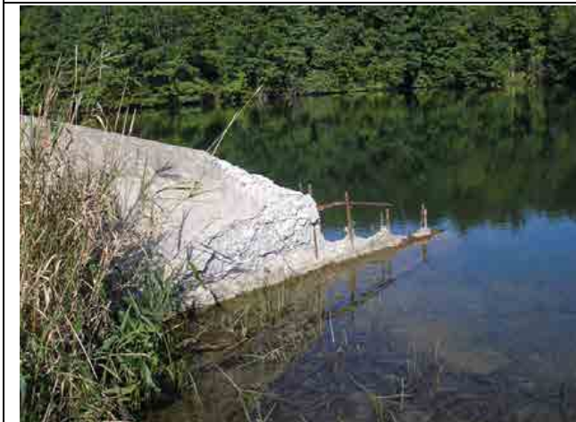
Photo #15 – Left upstream wingwall. Note missing concrete and exposed reinforcing bars.
