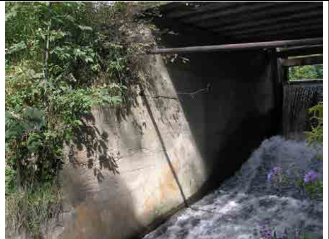
Photo #18 – Left downstream wingwall. Cold joint in concrete evident.
