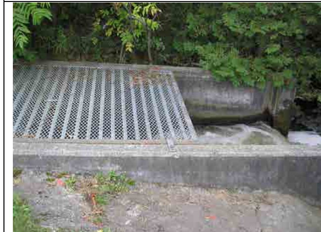
Photo #17 – Outlet of the fish ladder. Right bank is grouted with concrete. Opening in grate required for upstream fish migration. Opening poses safety hazard for staff.
