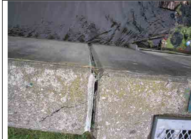
Photo #43 – Top view of the joint movement at the right downstream wingwall and fish ladder.
