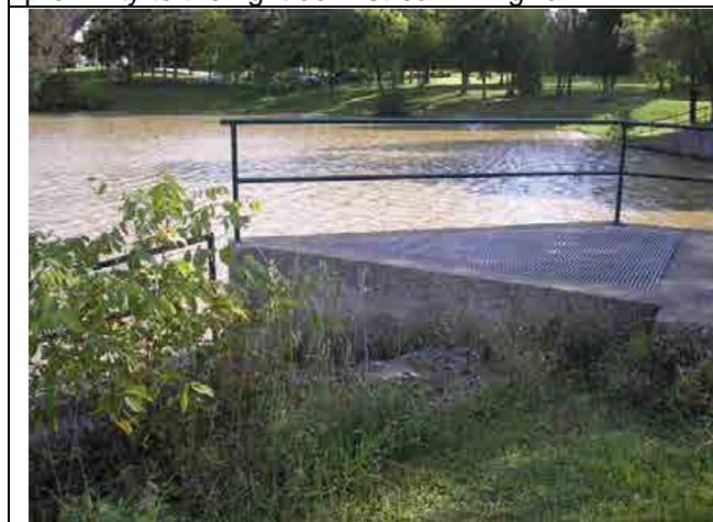
Photo #17 – Norwich Dam wetwell, located adjacent to the right wingwall on upstream face. Padlock on the steel grate noted as missing.
