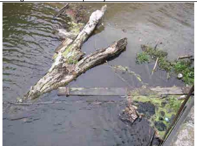
Photo #36 – Trash accumulation adjacent to the fish ladder intake gate.
