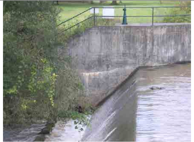
Photo #28 – Right downstream wingwall. Note signs of concrete deterioration.
