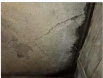
Image 27: Cracked foundation - Basement
