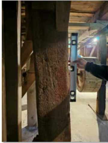
Image 13: Leaning Column - Basement
