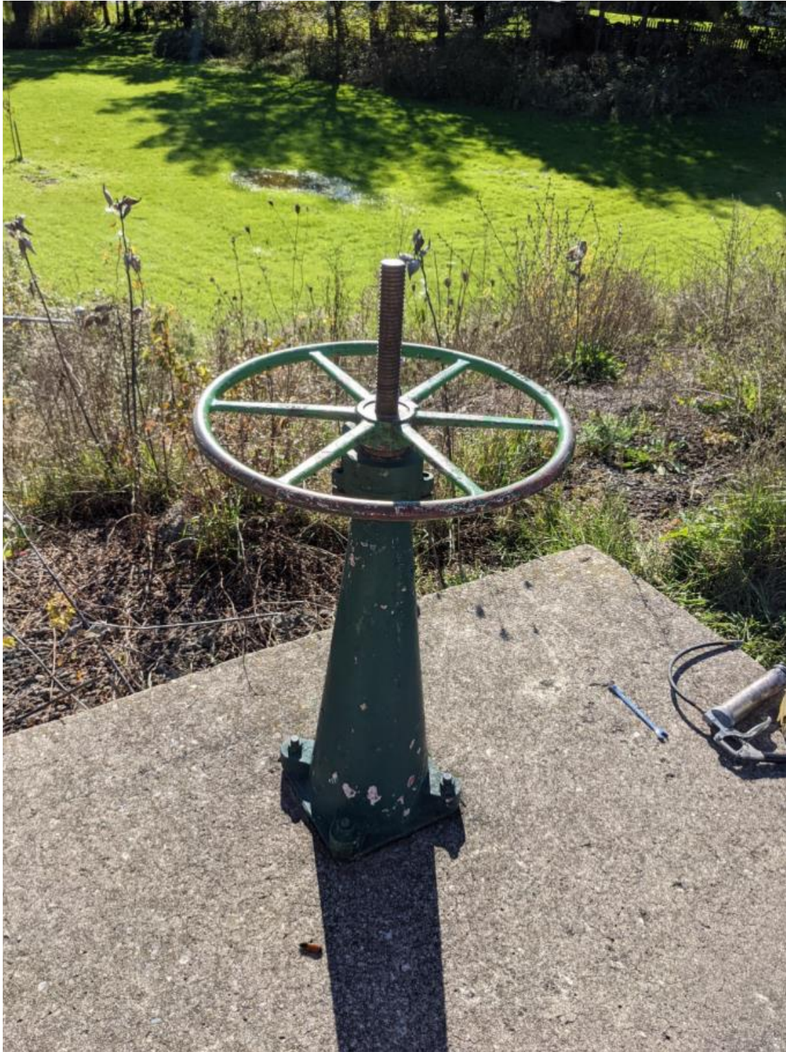
5. Low Flow Valve Control
